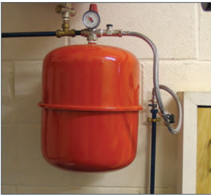
The expansion vessel and filling loop is usually positioned near the boiler.
