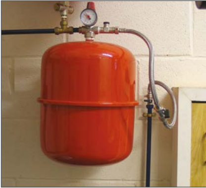
The expansion vessel and filling loop is usually positioned near the boiler.
